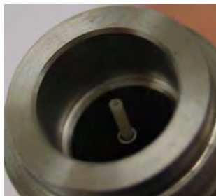
Sample line installed incorrectly
